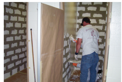
After experiencing difficulties filling mortar joints with an epoxy mortar, contractors applied Series 215 Surfacing Epoxy to achieve a smooth surface in the shower stalls at the Pine County Jail in Minnesota.
