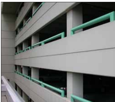
Series 157 Enviro-Crete, a flexible, breathable coating with excellent elastomeric properties, was chosen to protect the RSA Parking Garage in Montgomery, AL.
